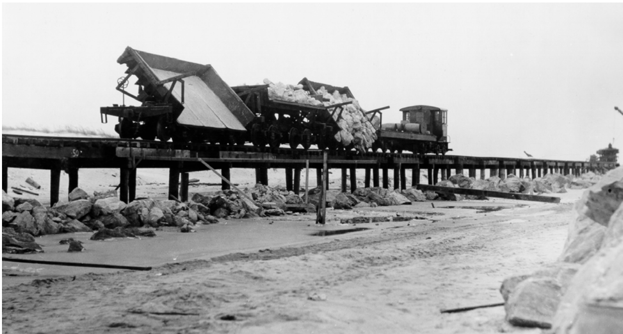
Figure I-3-6. Construction of Fire Island jetty on Democrat Point, at the west end of Fire Island, Long Island, New York. Many early USACE jetties were built from the land moving seaward using materials brought in by train. Photograph taken 3 Jan 1940, from Beach Erosion Board Archives.
