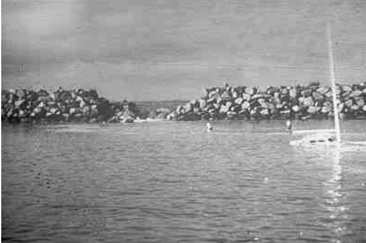
Figure VI-8-6. Damage at Redondo Harbor breakwater looking from inside harbor (circa 1988)
