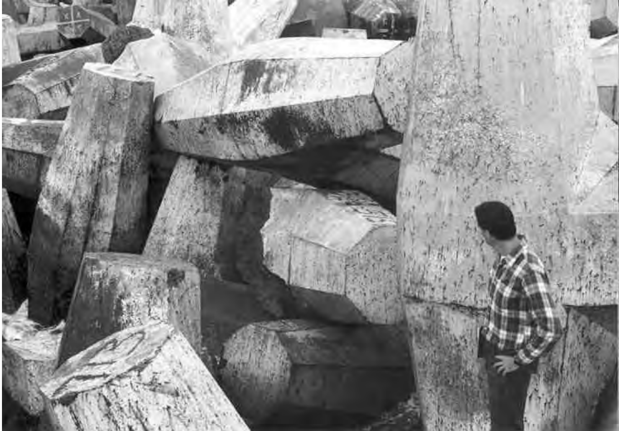
Figure VI-8-1. Dolos breakage on Crescent City, California, breakwater
