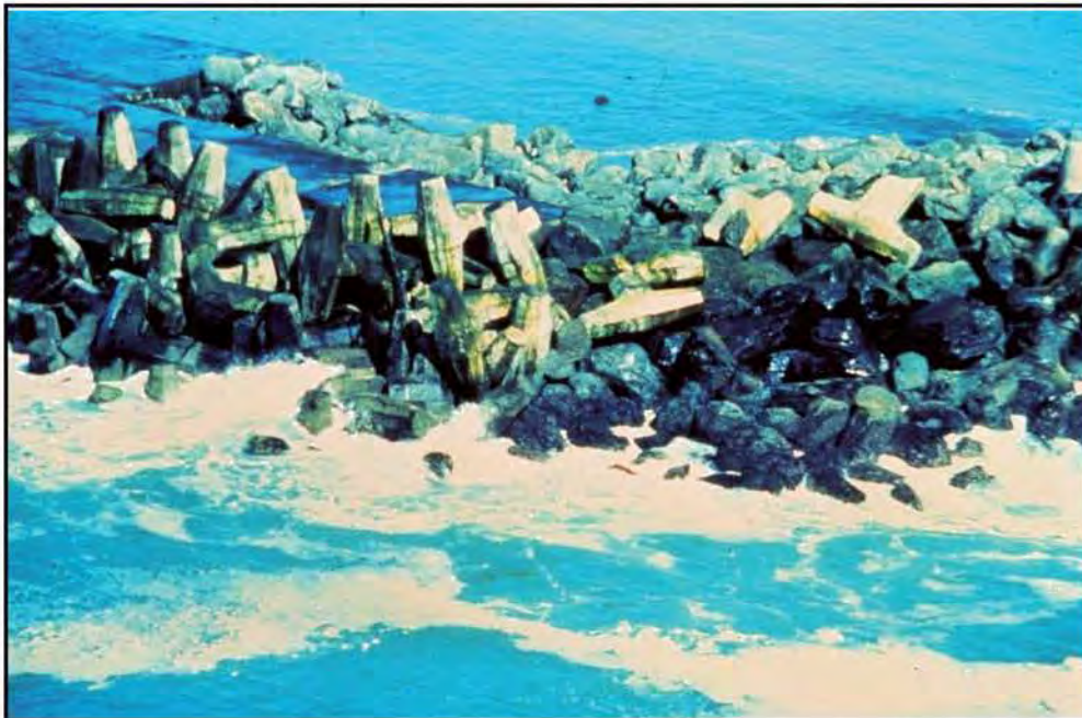
Breakage of armor units
