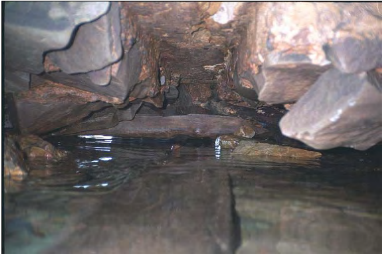
Looking along Interior Centerline of Great Sodus East Breakwater Parapet, Lake Ontario, New York
