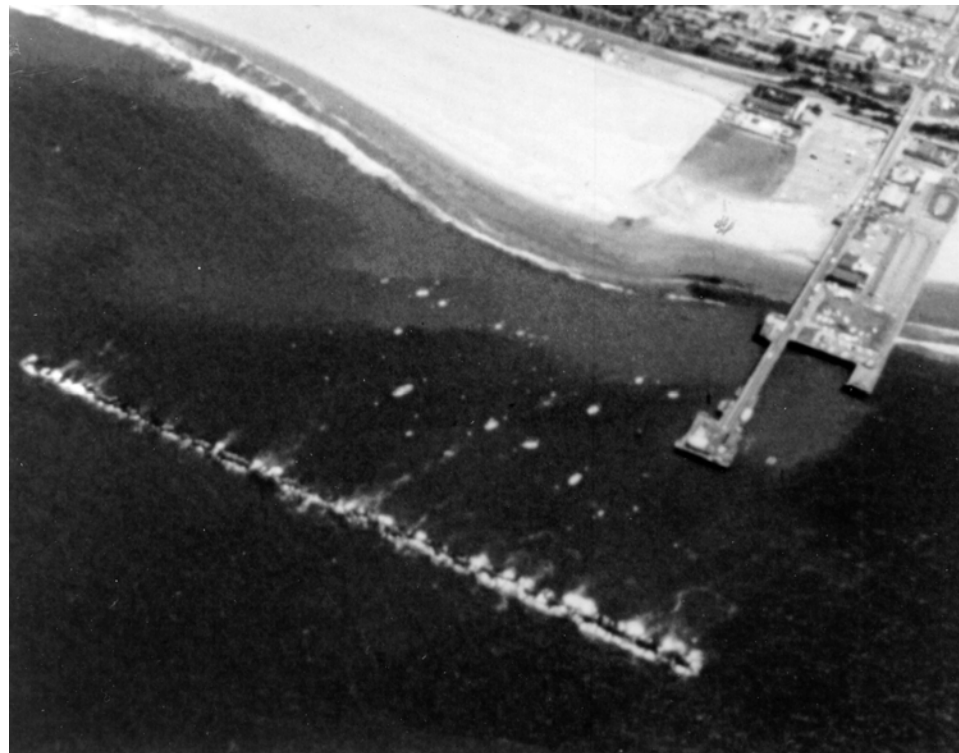
b. Deteriorated breakwater allowing wave transmission
