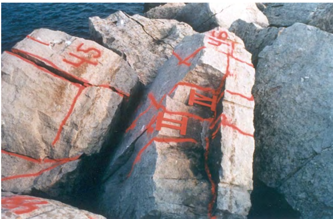
Figure V-2-12. Cracked dolomitic limestone - Cleveland East breakwater, Ohio, 1989 (stone is dolomitic limestone)
