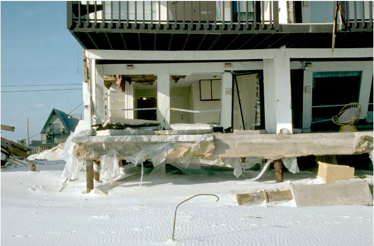
Figure IV-1-14. Hurricane Opal damage at Navarre Beach, Florida, November 1995. The sand underneath the concrete slab washed away, and the unsupported floors collapsed
