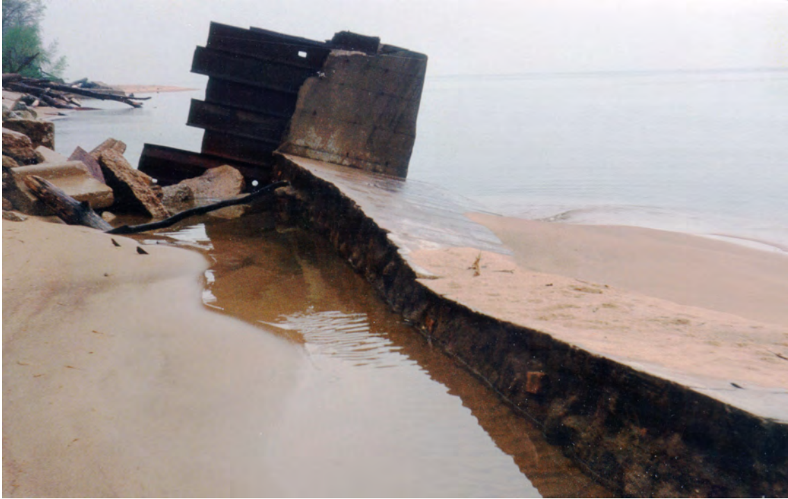
Figure III-5-27. A toppled concrete seawall along the Lake Michigan coast of Berrien County. Failure probably resulted from undermining of the underlying glacial till foundation, April 1991
