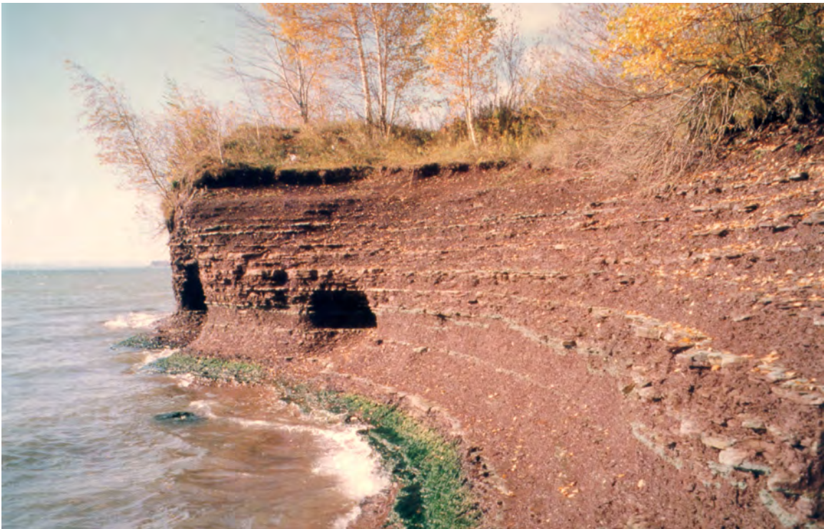
Figure III-5-23. An eroding shale bluff along the west Lake Ontario shoreline
