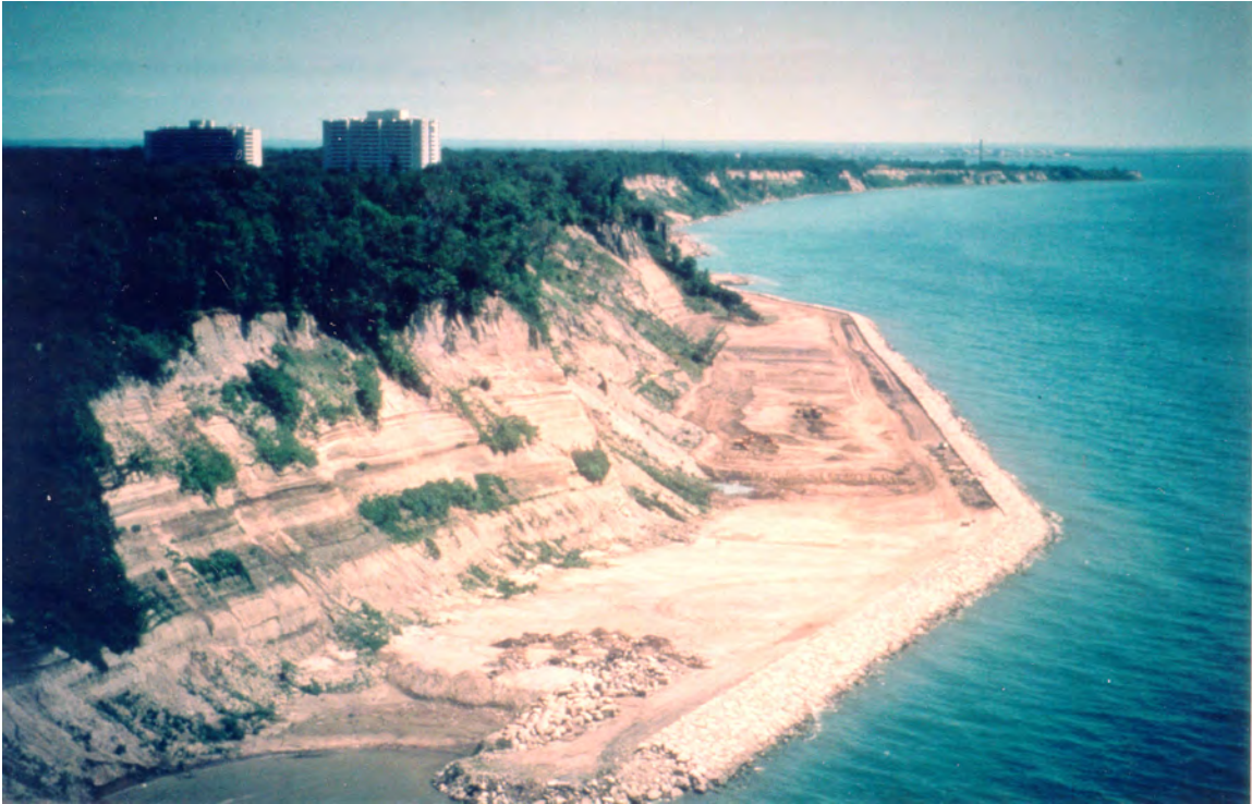
Figure III-5-24. Shore protection consisting of a wide berm protected by a revetment along the base of the Scarborough Bluffs located east of Toronto on Lake Ontario
