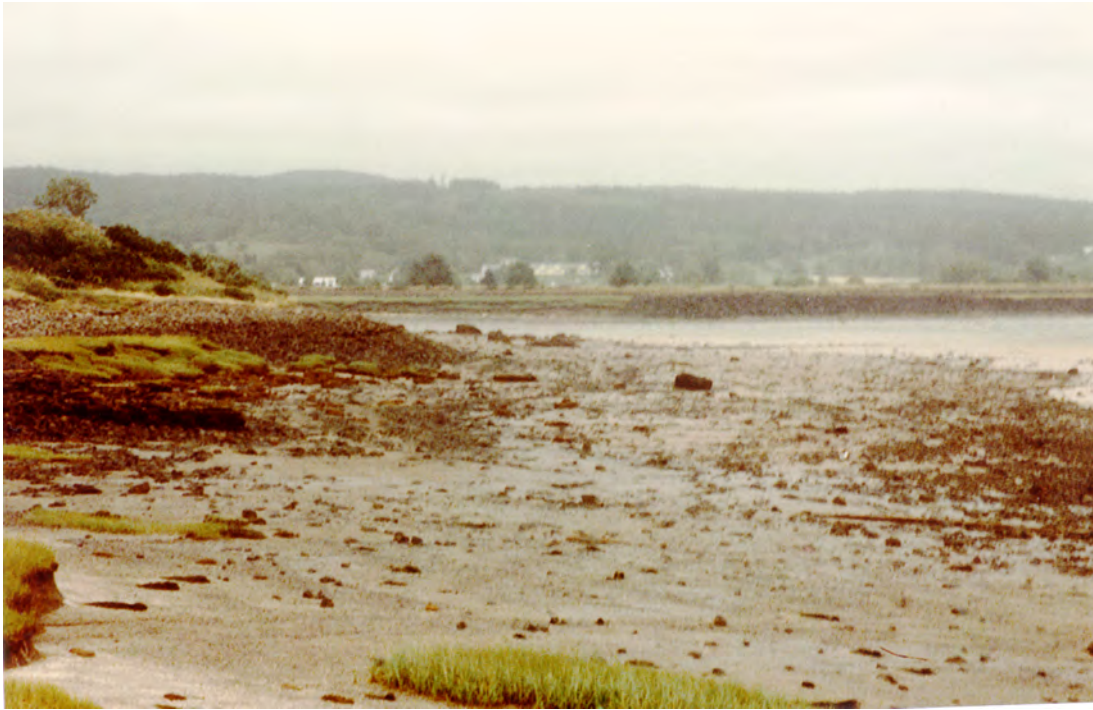
Figure III-5-8. A mud 'beach' backed with eroding salt marsh at Annapolis Royal, in the Annapolis Bay of the Bay of Fundy. Basalt revetment at top of salt marsh is an attempt to halt the erosion
